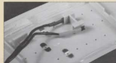
Accessory wire with female quick connects attached to FasTrack electrical terminals
